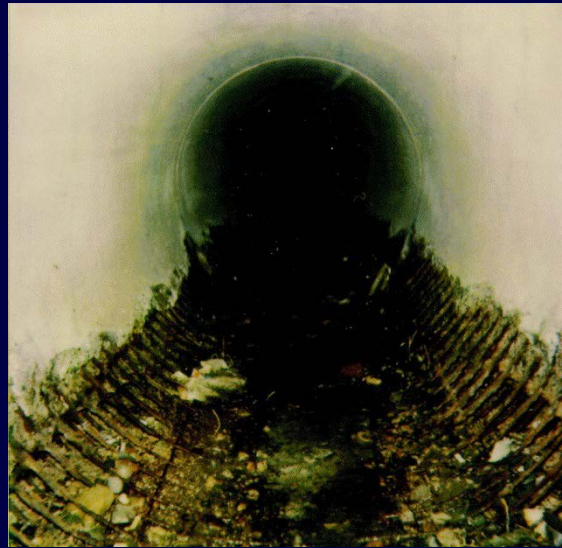
Acidic factory discharge, I-94 St. Paul Metro District
