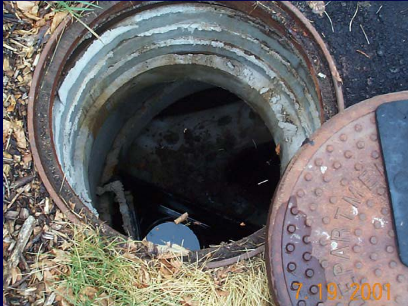
Manhole (solid cover) with too many rings
